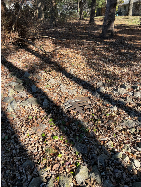
Upstream drainage structure with CPP submerged in water.
