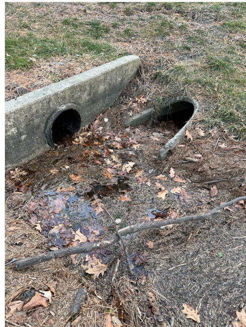
12" CPP with concrete headwall. Pipe recently cleared of debris according to HOA.
