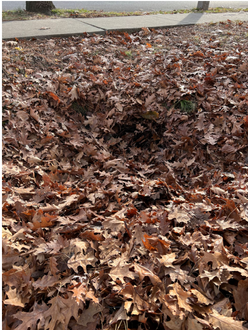
12" concrete pipe @ Smyth Dr clogged with leaves causing water backup and long-term ponding.
